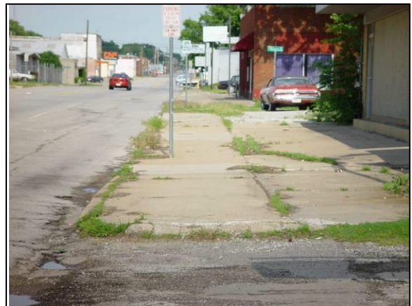
• Figure 23 Aging infrastructure is a key concern.
